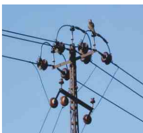
Electric pole for electricity
